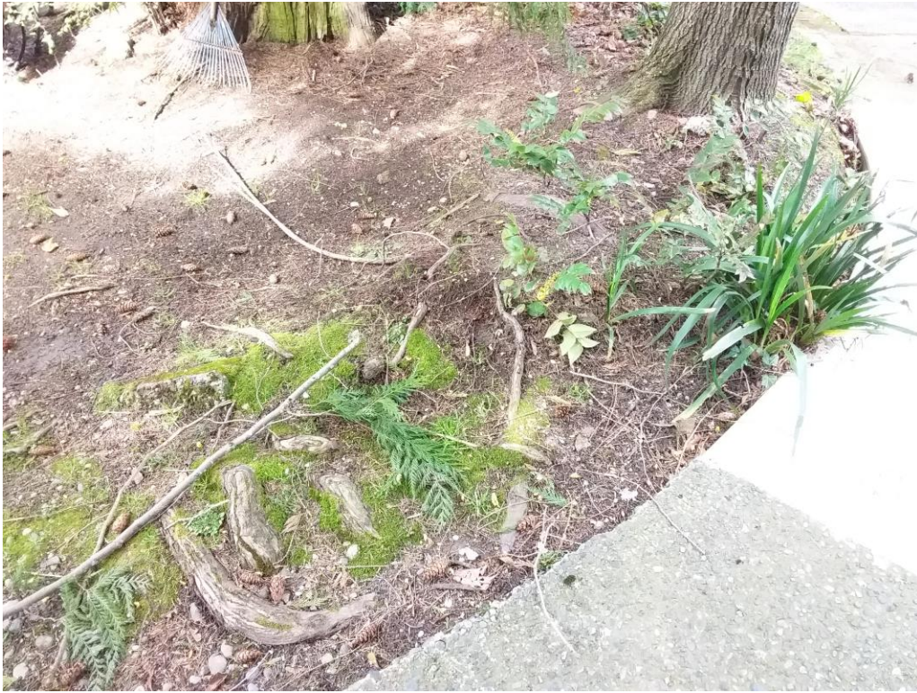
Figure 48. Roots of the #30 cedar pushing up against the driveway.
