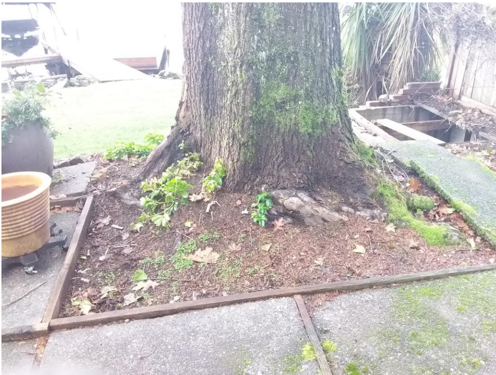
Figure 16. Looking west at the base of the #1 oak showing uplift of patio.
