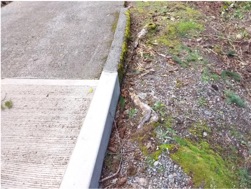
Figure 43. One of the #19 cottonwood roots pushing up against the entry drive curb.
